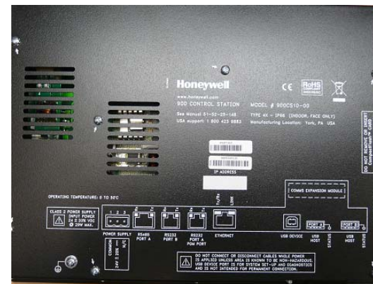
Power and Port Connections
